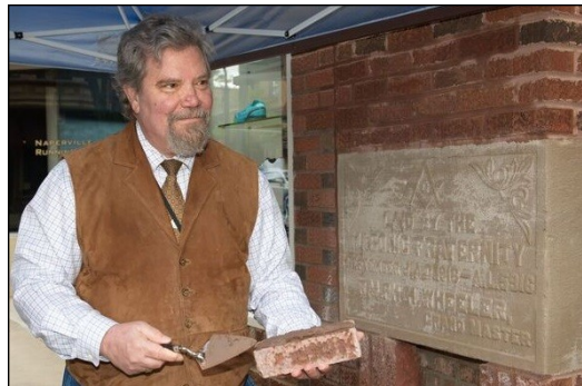
WM Ingraffia spreading the cement on one of the bricks used to seal the time capsule in the cornerstone
